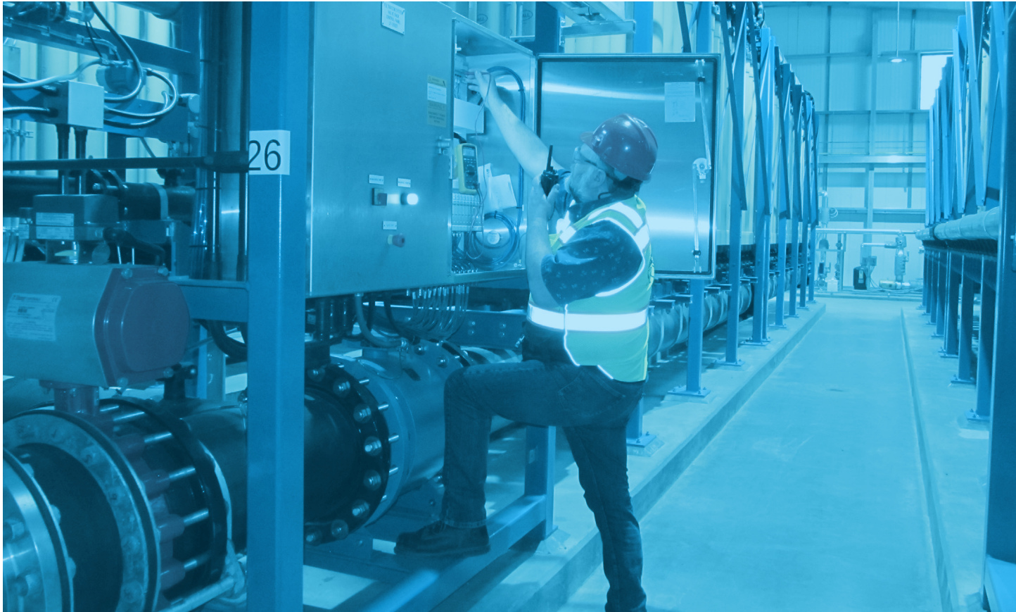
Spokane water reclamation facility
