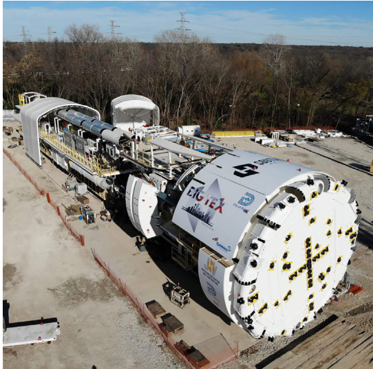
The project will provide 100-year flood relief for 2,200 commercial and residential properties. Here, the "Big Tex" TBM is assembled above ground in preparation for deployment.
