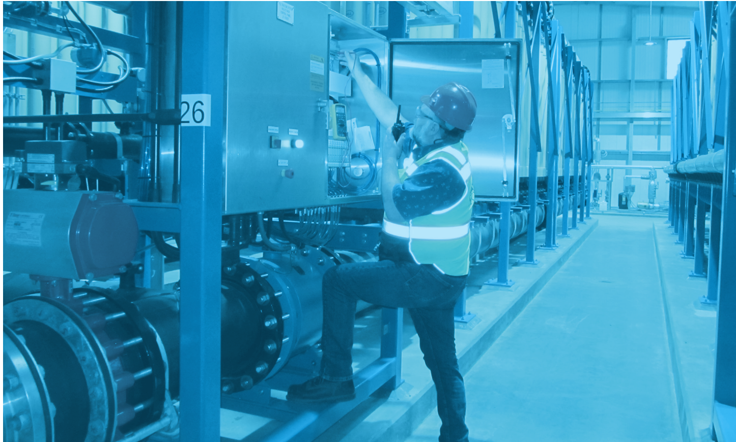
Spokane water reclamation facility
